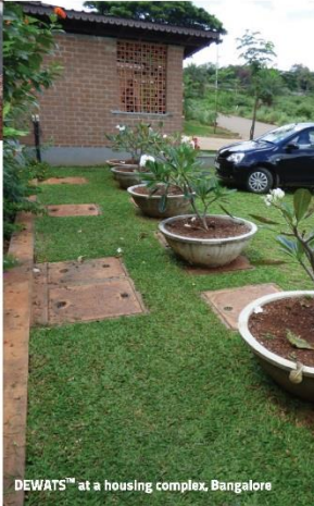
DEWATS™ at a housing complex, Bangalore
